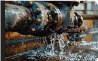
Situation: LEAKING OF OIL, AIR, WATER
