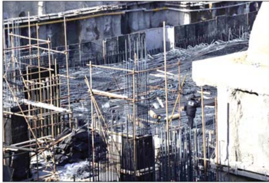
Concrete slab collapse
