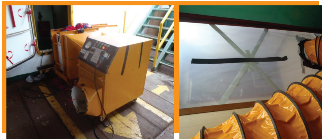
Figure 6.4: Air pump to maintain air change per hour
