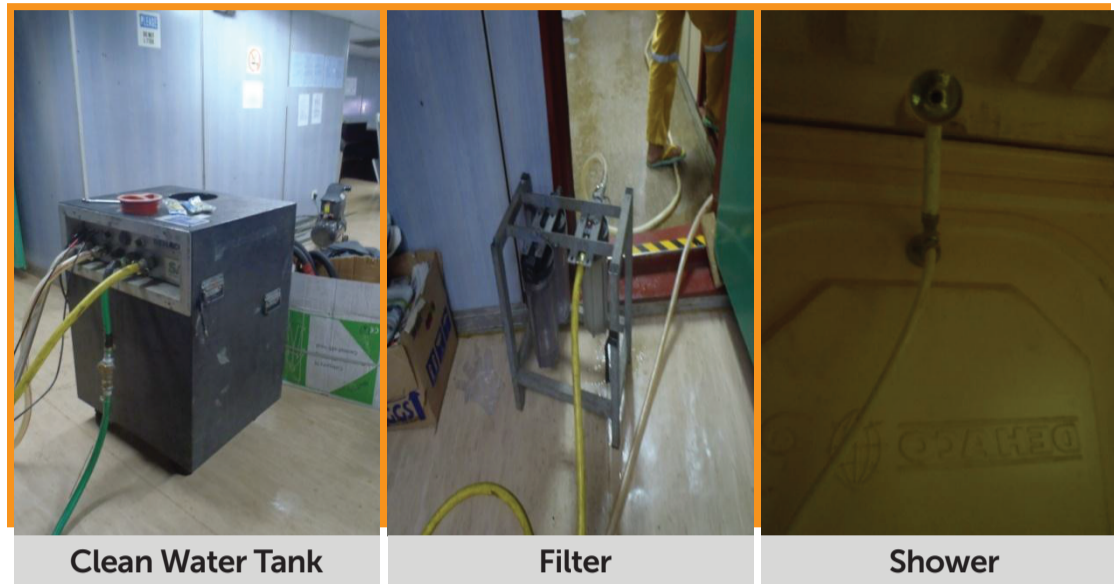
Figure 6.6: Example of shower facilities
