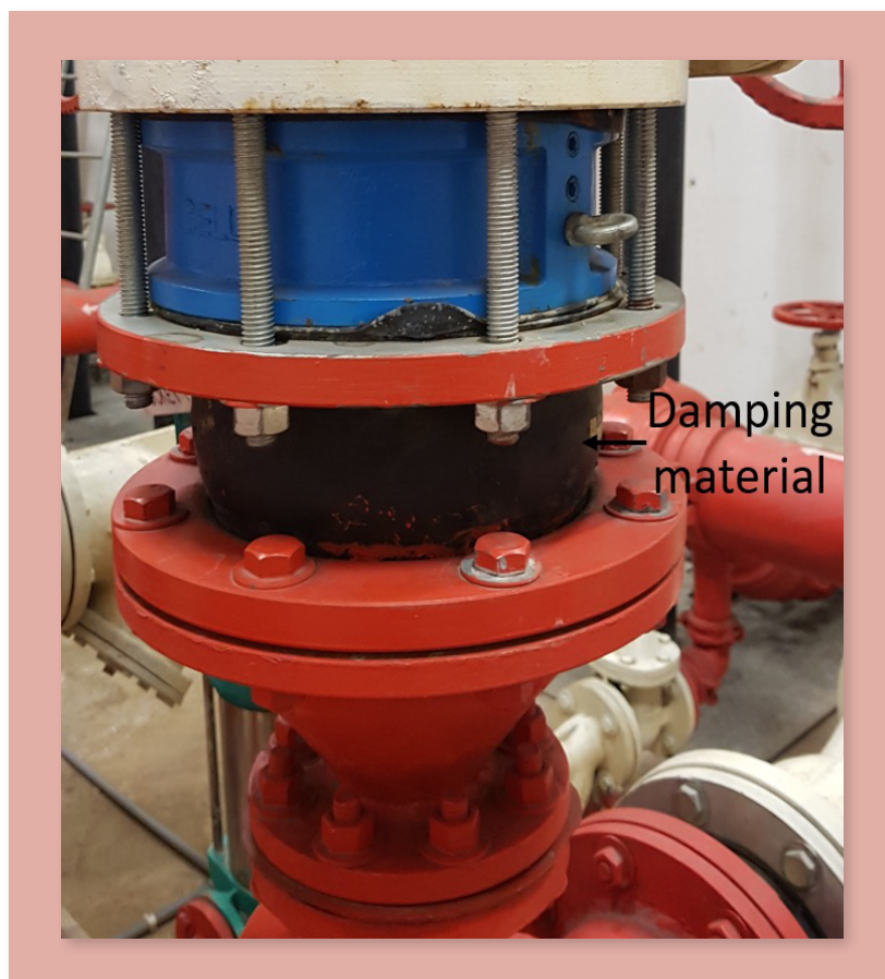
Figure 6.29: Damping material located between two steel pipe connections.
